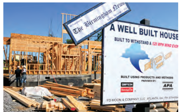
This sign describing building methods that can withstand 120-mph winds is placed in front of a home in Pratt City. The house that originally stood on this spot was destroyed on April 27, 2011, when a string of deadly tornadoes struck Alabama.
